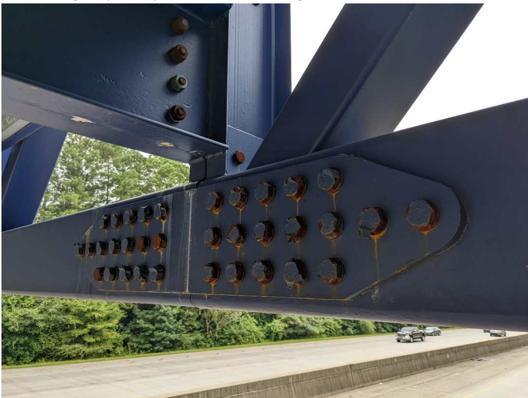
Photo 4 – Typical damaged to protective coating
