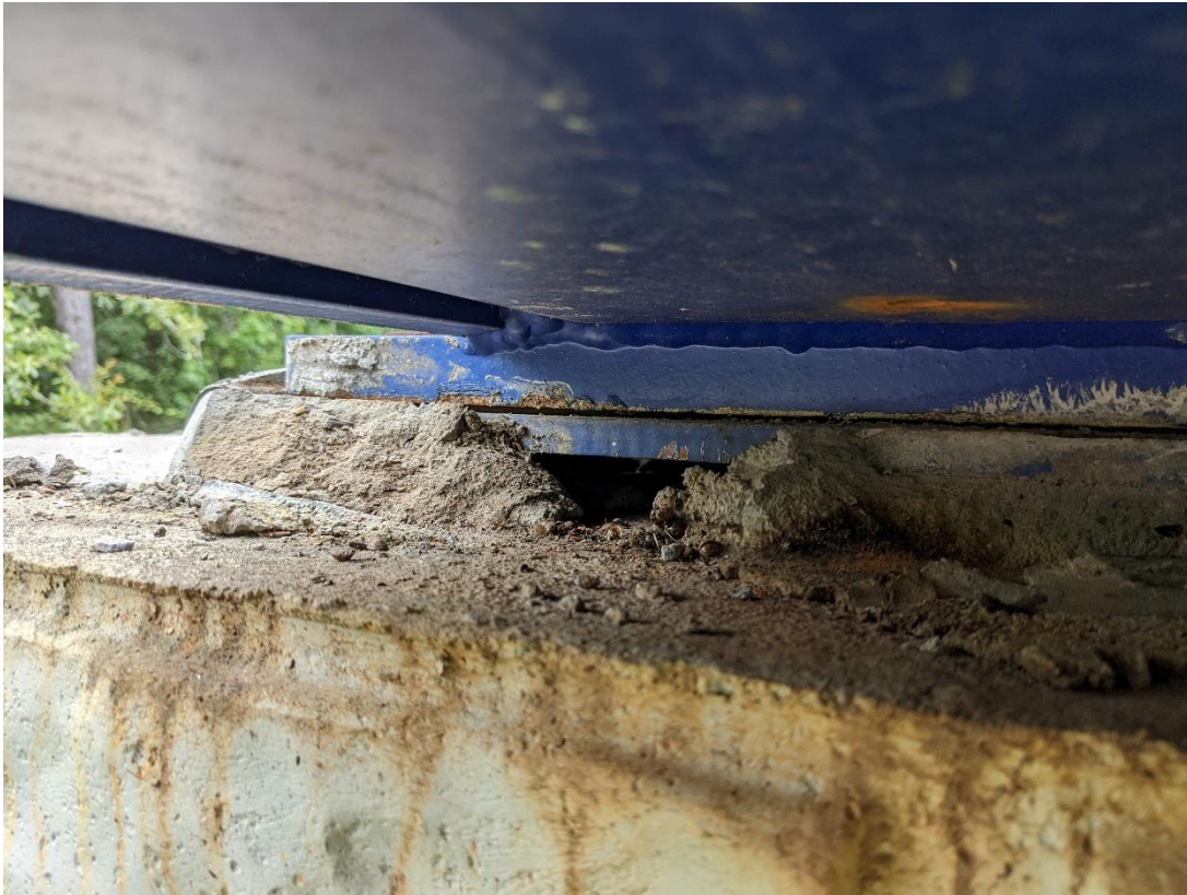
Photo 3 – Void in grout pad at Span 2, Bent 3, left bearing
