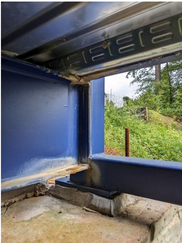
Photo 6 – Evidence of water intrusion
