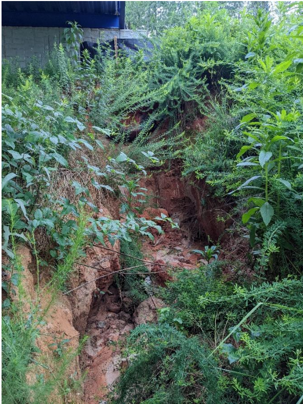
Photo 5 – Erosion of slope at Bent 1
